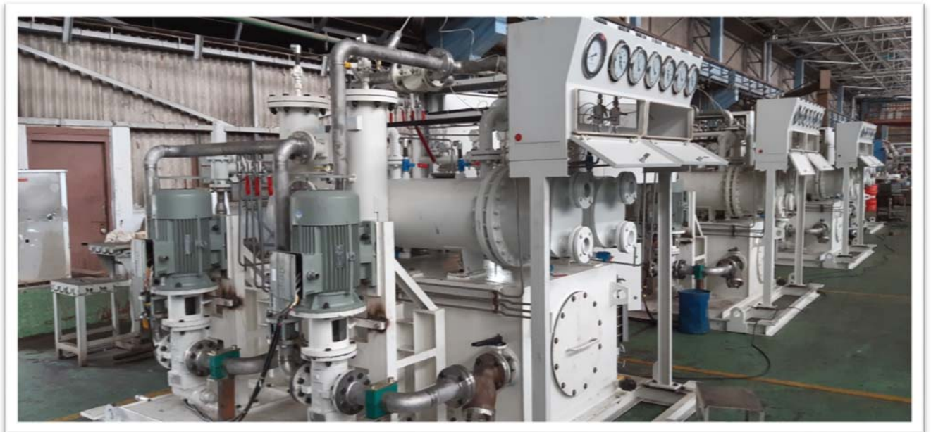
Lube oil systems under testing
